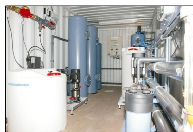
An example of a custom-designed permanent solution with dosing, softening, carbon filtration and reverse osmosis
